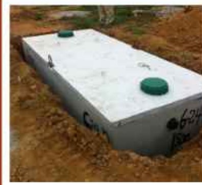
COMMON SEPTIC TANK
