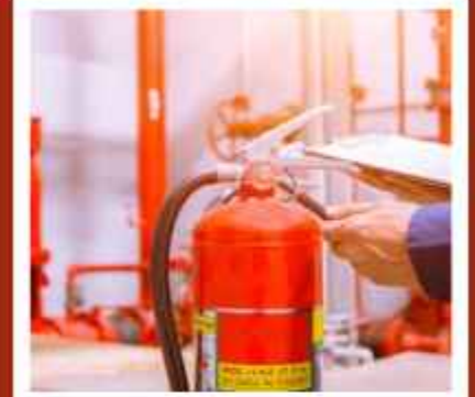
FIRE FIGHTING SYSTEM IN CLUB HOUSE
