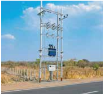
DP FOR ELECTRICITY CONNECTION
