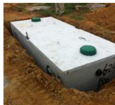
COMMON SEPTIC TANK
